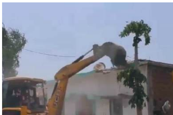
A bulldozer demolishes a home in Bhainswahi Village in Madhya Pradesh. Photo via The Observer Post.
