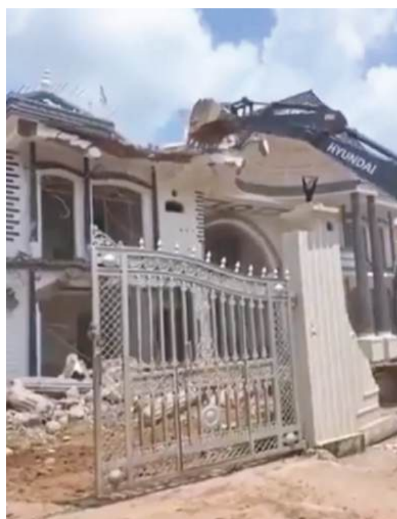
A bulldozer demolishes the home Muslim leader Shehzad Ali in Madhya Pradesh.
